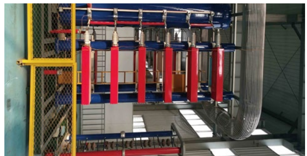
Lightning impulse voltage generator
