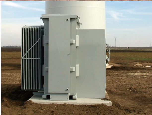
USA 3150KVA Wind power pad mounted transformer
