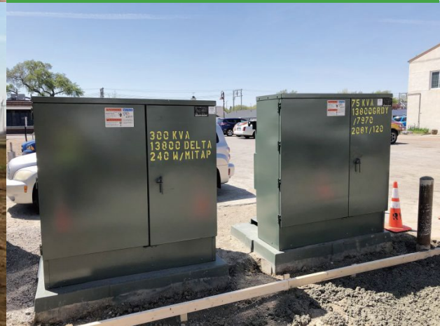
Guyana 300kva pad mounted transformer
