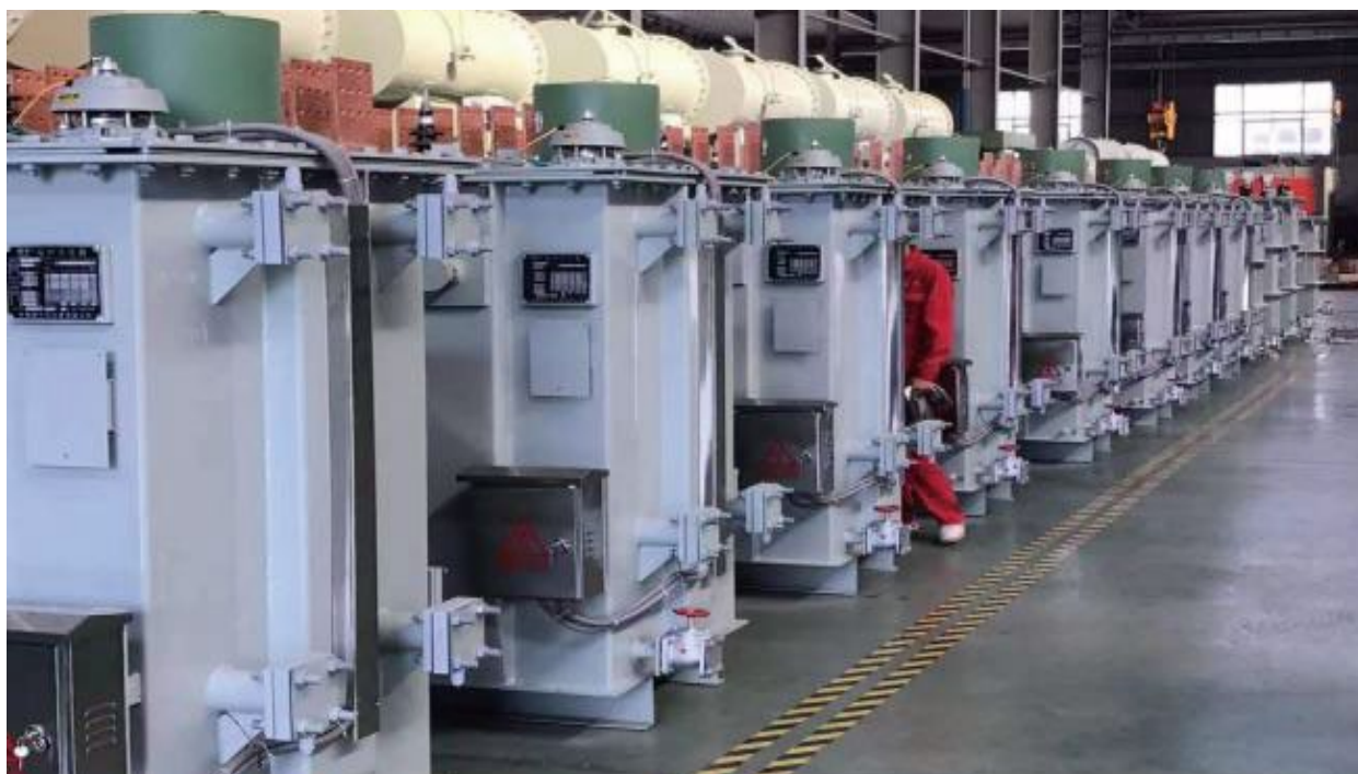
▲ 10kv furnace transformer
