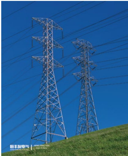
Lattice Steel Tower
