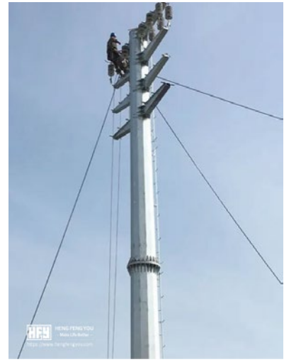
Steel Pole Tower
