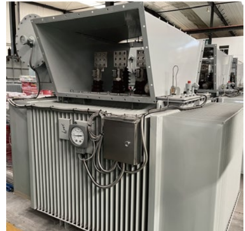
20kV/3mva oilfield specific transformer
