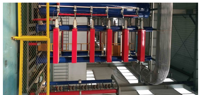
Lightning impulse voltage generator
