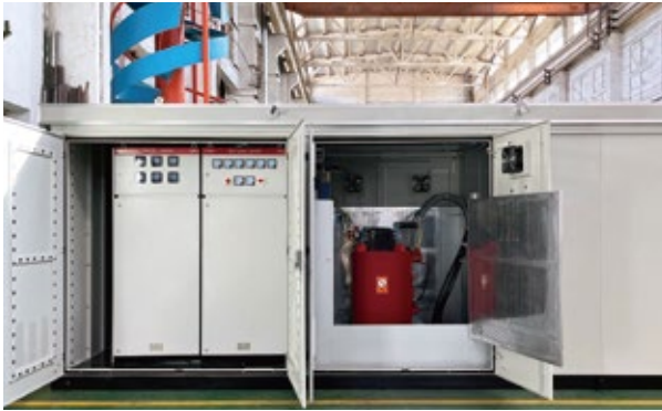
▲ 800KVA DRY TRANSFORMER COMPARTMENT
