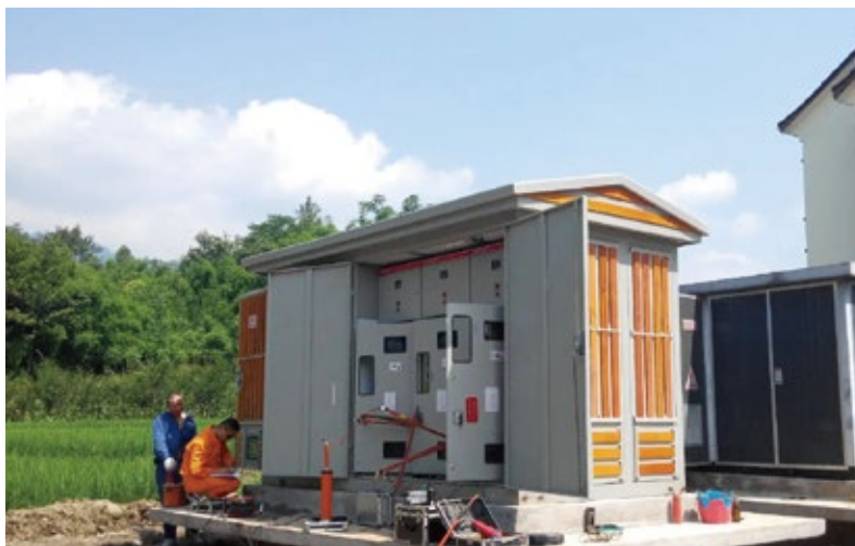
▲ Installation site of landscape Compact Substation
