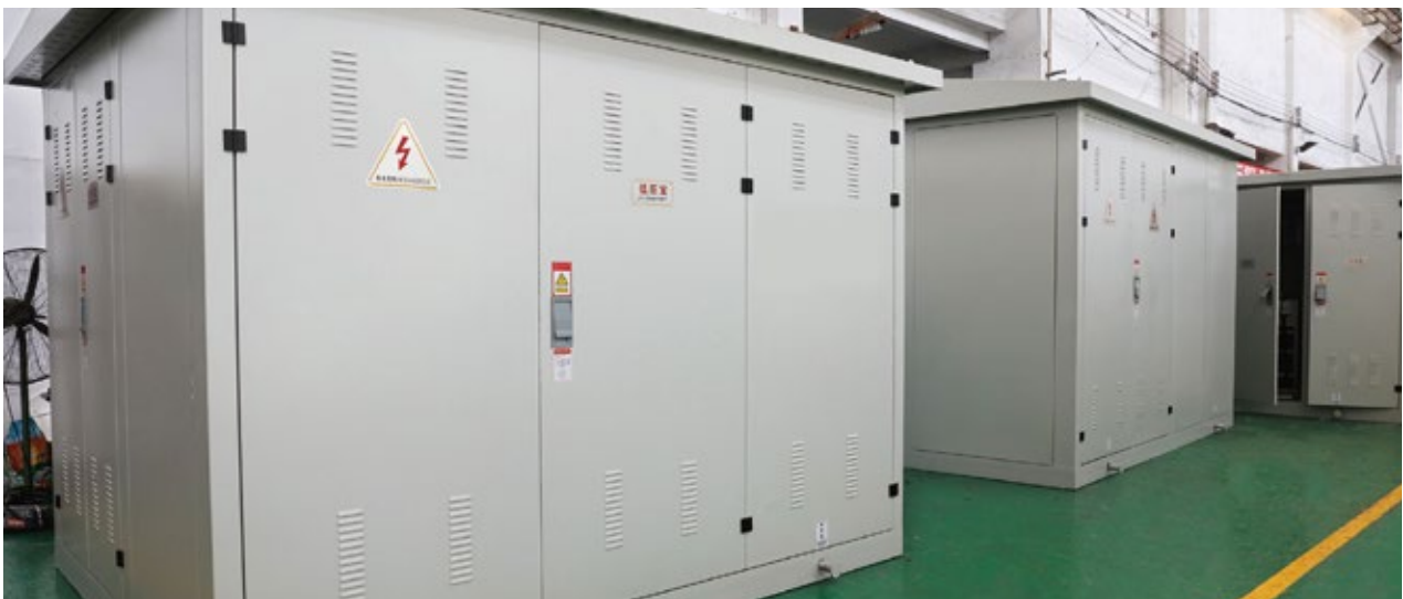
▲ SUBSTATION FOR SOLAR POWER GENERATION
