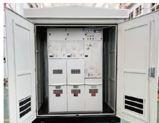
>High voltage room-800KVA
